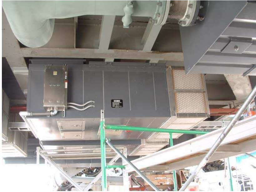
Figure 5: One of the 12 Acoustical Inlet Hoods under the CT with filtered air inlets
